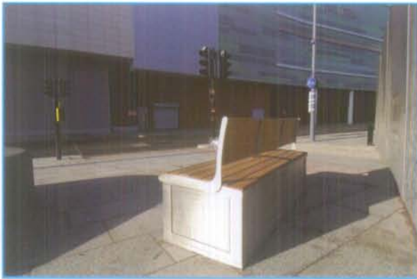
Bench containing traffic signal controller
