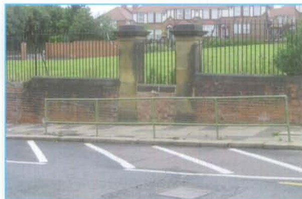
This guardrail has no function - the pedestrian route it was protecting has been closed - and can therefore be removed.
