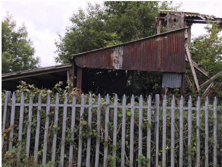
Photo 67: Looking west from Lords Lane at dilapidated building
