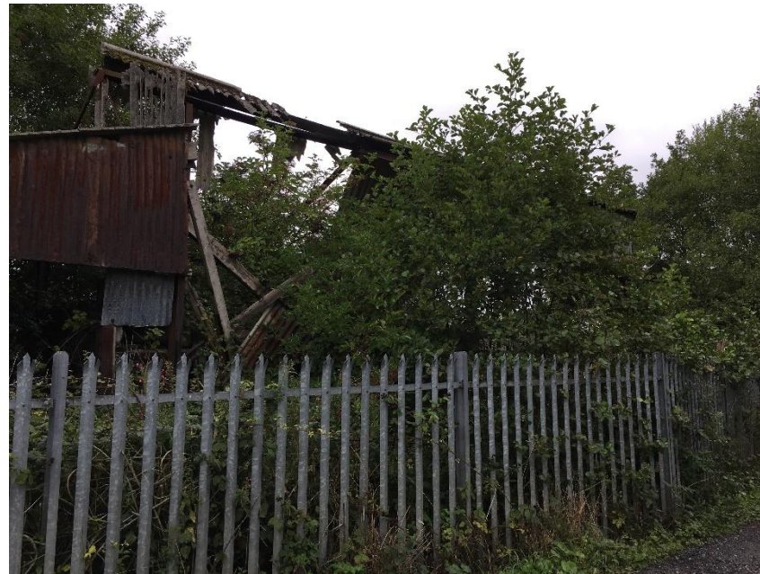
Photo 68: Looking west from Lords Lane at dilapidated building
