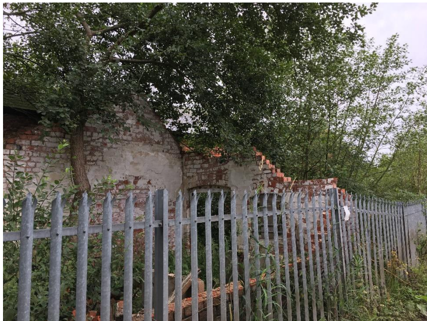
Photo 70: Looking west from Lords Lane at dilapidated building
